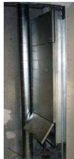
Fig. 1.2. Heat recovery unit from EcoVent placed in a small technique room in the dwelling.
