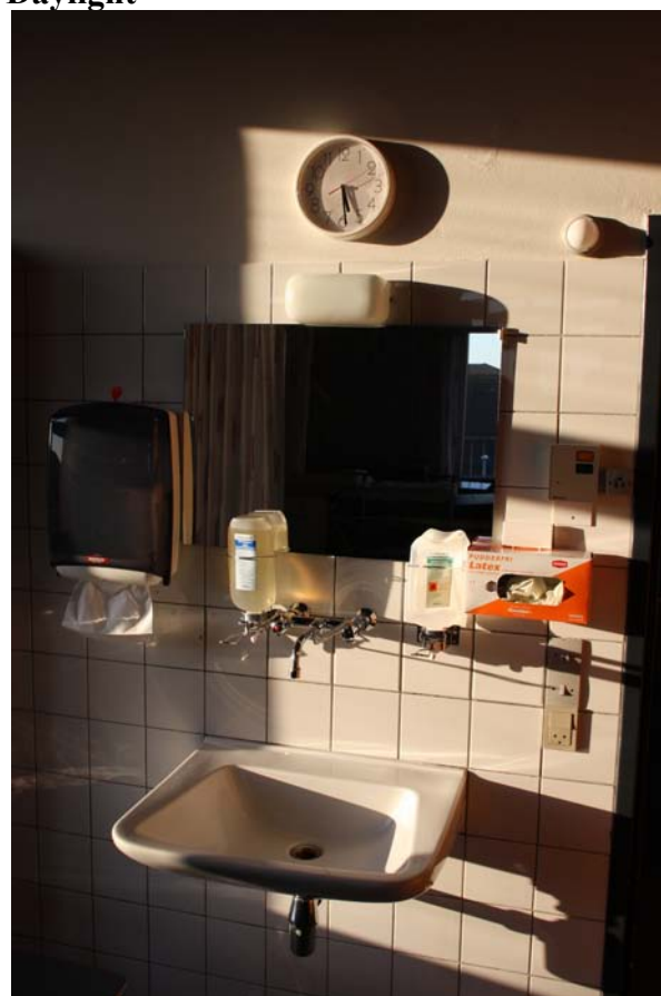
Figure 17: Hospital sink in daylight
