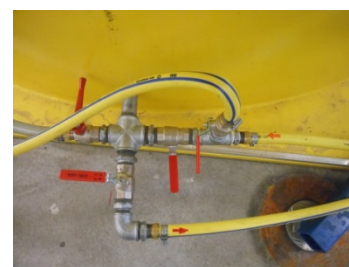
Figure 2. In and out flow valves.
