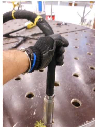
Figure 9. Vibration starts inserting the rod vibrator in the hole marked in yellow.
