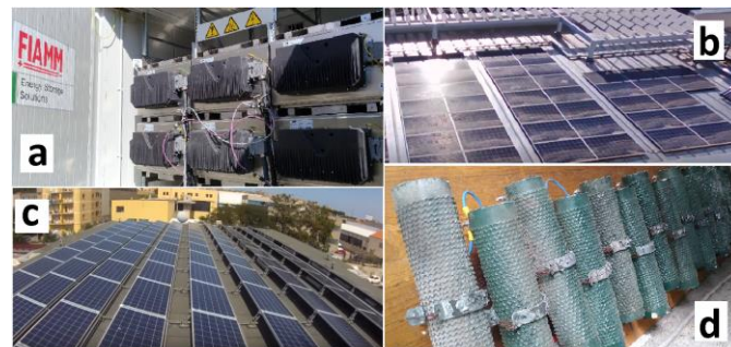
Fig. 4. a) FIAMM storage; b) PV1 generating unit; c) PV2 generating unit; d) adjustable load
