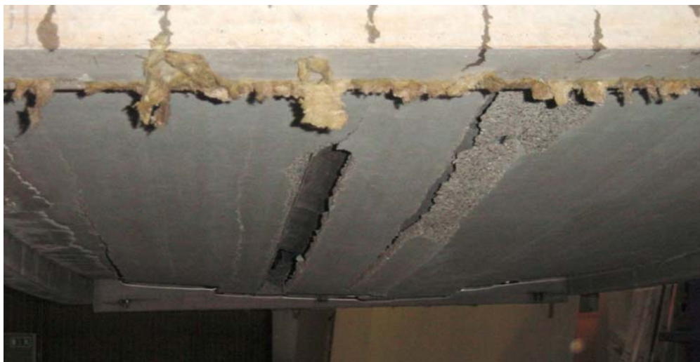
Figure 8. Damages after 25 minutes. Photo K. Hertz.
