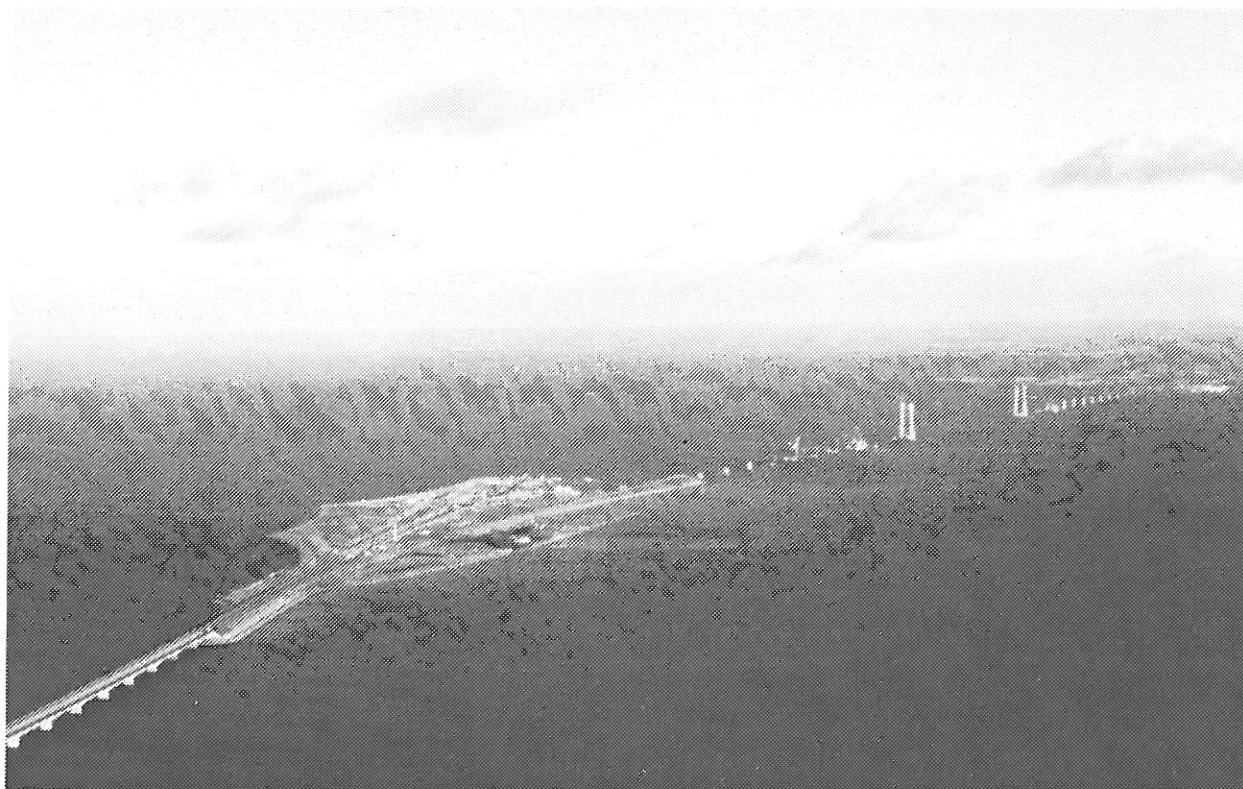
Fig. 3. View of Storebælt Link project in late 1994. The West Bridge is in the final stage of fitting; the cut and cover parts of the tunnels on Sprogø and in Halskov are almost completed and one of the twin tunnels are open for passage (Photo by J.K. Winther)
