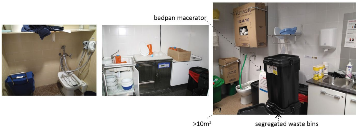
Figure 16. Dirty utility room at HCUV, HD and HUV.
