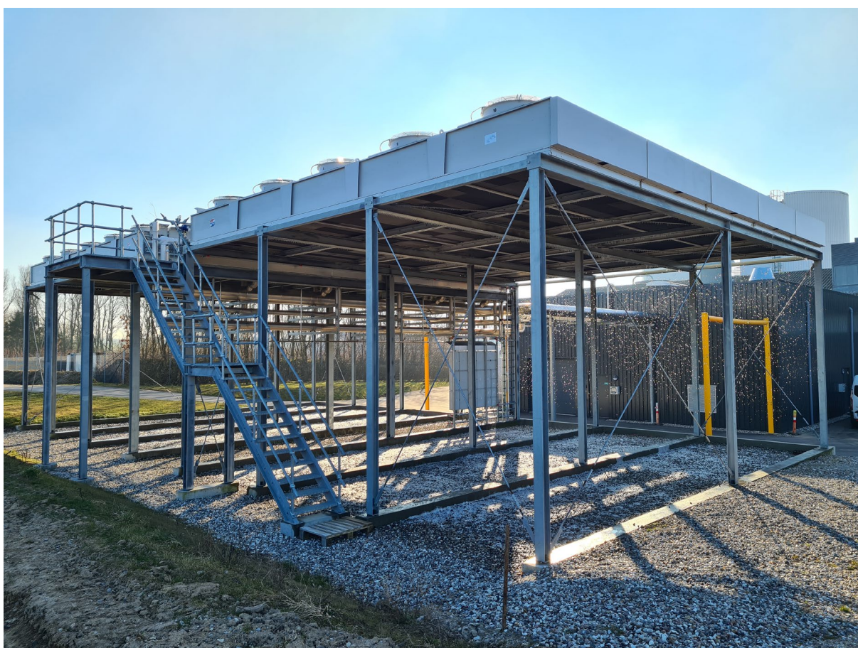
Figure 5: Flatbed air coolers of the 3 MW heat pump at Præstø Fjernvarme, Denmark; source: Daniel Trier (PlanEnergi).
