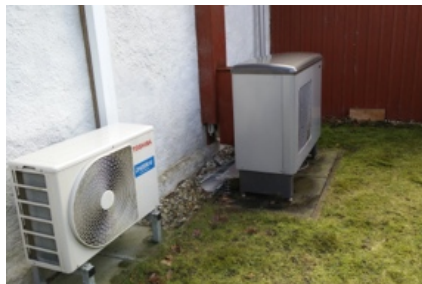
Fig 4: An air to water heat pump at one of the participating households.
