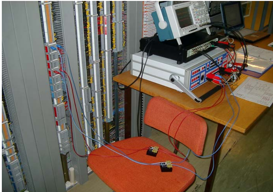
Figure 5.19 The values were measured as a voltage drop on low-inductance resistors, using the Omicron CMC256 unit and B&K 24bit data acquisition unit.
