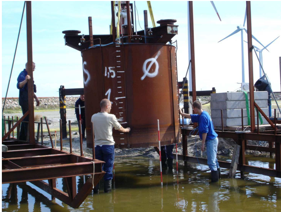
Figure 10: Field tests of installation and bearing capacity of a bucket foundation with d = 2 m and D = 2 m, Frederikshavn 2002
