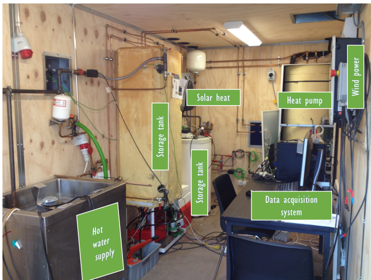
Fig. 25: Experimental set-up used for hot water tank model validation
