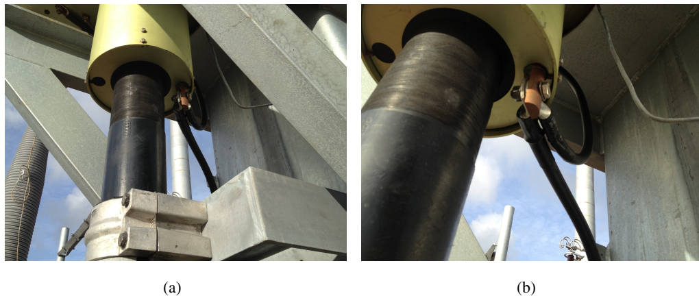
Figure 7.10: Extraction of cable sheath at cable termination.
