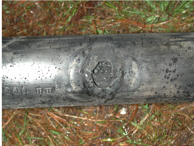
Figure 1.2: Fault on a single-core cable used for the Horns Reef 2 connection.
