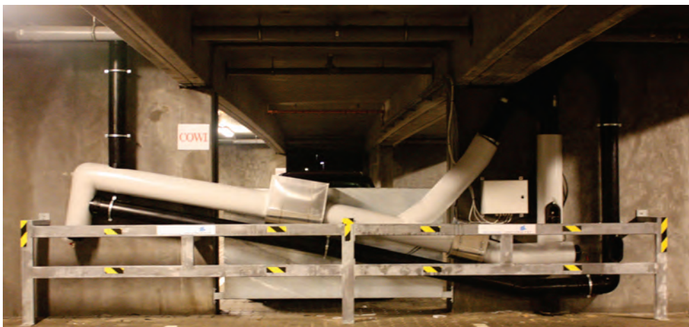
Figure 16: The runoff measurement system with heating cables, insulation and collision protection.
