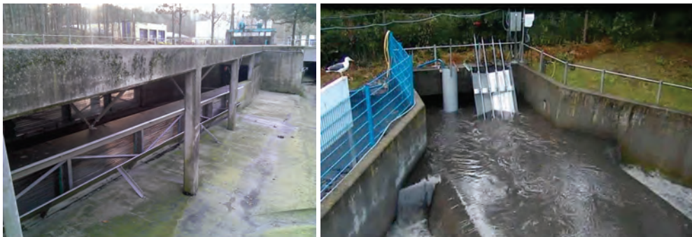
Figure 23: Photo of the internal CSO during dry and wet weather. The photos are taken from the northerly side of overflow structure towards west and east, respectively. The overflow structure are symmetric along the centreline of the inflow channel.
