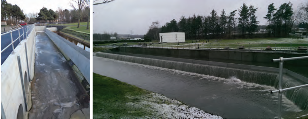
Figure 24: Photo of the external CSO during dry and weather. The photos are taken from the westerly and south-easterly sides of the overflow structure, respectively.
