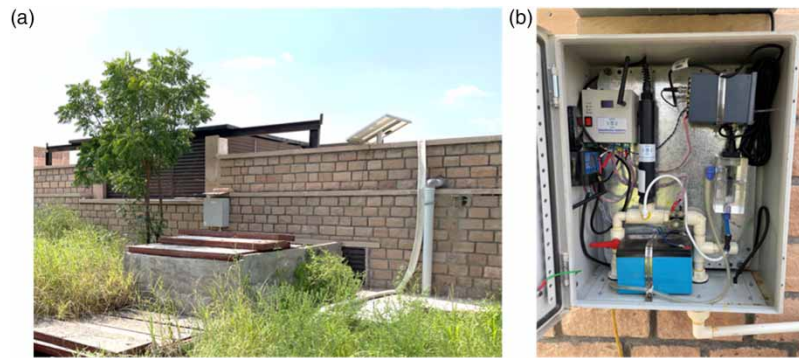
Figure 6 | Quality node and its components. (a) Above the ground unit with solar panel. (b) IP67 enclosure for housing IoT devices and other components.
