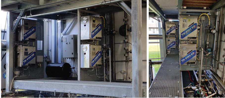
Fig. 2.9: Photos after installing four OiW monitors with two monitors on each sidestream. The sampling probes are installed in a vertical pipe section with flowmeters and control valves to maintain a constant flow rate through the monitors.
