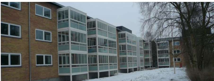
Figure 4. Photos of the old facade (top), new facade before the balconies were mounted (middle) and the new balconies (bottom).
