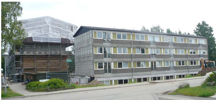
Figure 1. Two of the three blocks at Traneparken. The photo shows the end wall of one block being renovated and the facade of the other which has not yet been renovated.
