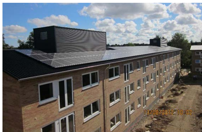
Figure 2. The 33 kWp south-facing PV system and the coverings for the new mechanical ventilation systems located above each stairway.
