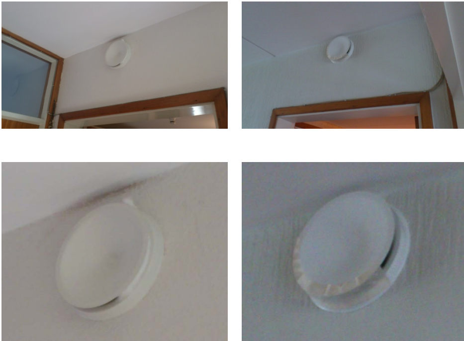
Figure 5.7. Examples of supply air terminals with partly blocked openings due to draught.
