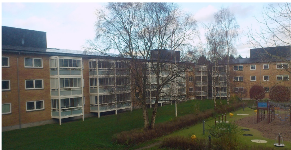
Figure 5.1. The ventilation units are housed in custom made shelters placed on the roofs of the buildings.
