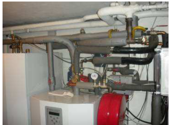
Fig. 4. Typical heat pump installation from the IFIV project.
