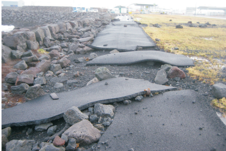
Figure 1. Example of damage due to heavy overtopping. Photo from a walkway at Ananaust, Reykjavik, Iceland. Due to overtopping the pavement has been damaged and rock fill behind the structure has eroded.
