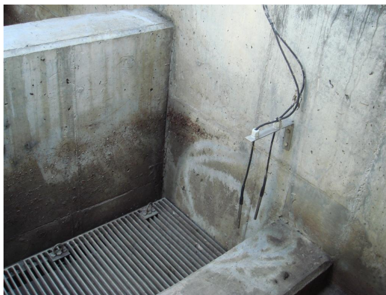
Figure 4. Water level switch for overflow indication
