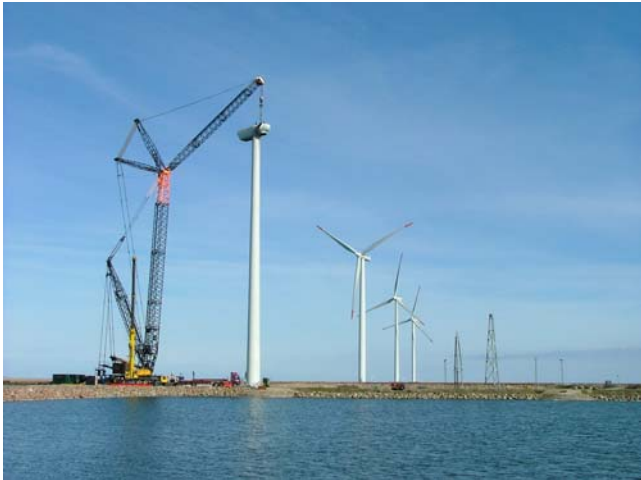
Figure 19. Replacement of nacelle in the spring 2005. The four wind turbine at the test field in Frederikshavn is shown. The Setup for combined loading of 2x2m bucket is also shown.
