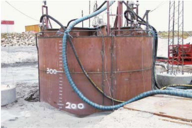
Figure 11. The critical suction has been achieved and soil failure by piping has occurred.
