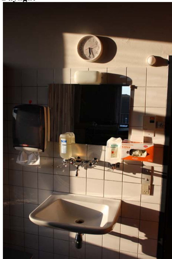
Figure 17: Hospital sink in daylight
