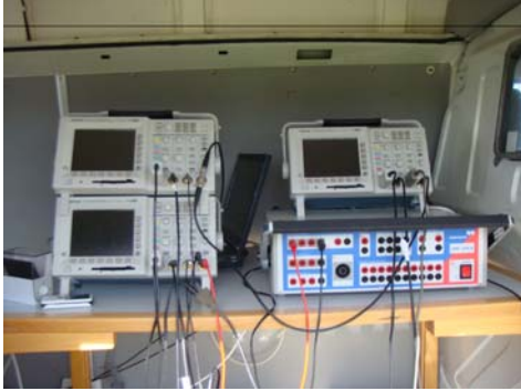
Fig. 7 Measurement instruments for cable measurements on 400 kV cable
