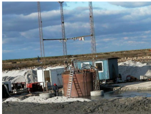
Figure 1. Installation tests on 4 \times 4 m buckets in a natural seabed at the test site in Frederikshavn, Denmark.
