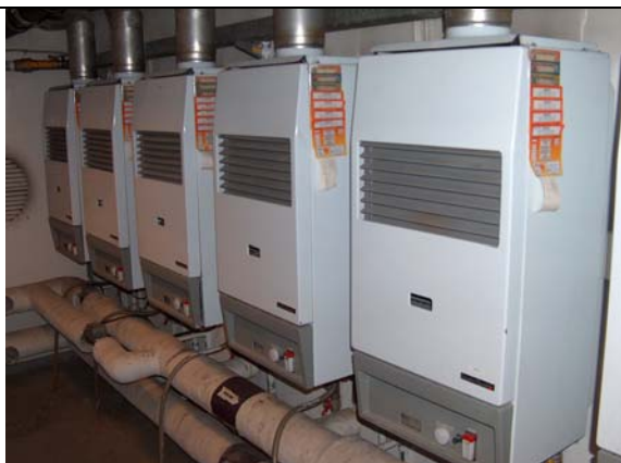
Natural gas boilers operating in cascade.
