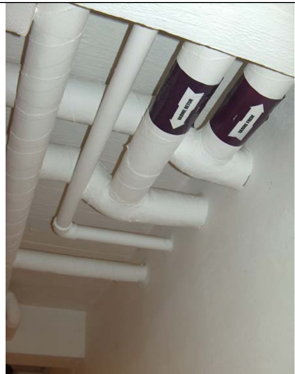
Insulated heating distribution system in basement.
