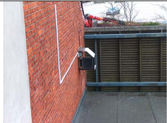
Wall mounted condenser for cooling engine for canteen.
