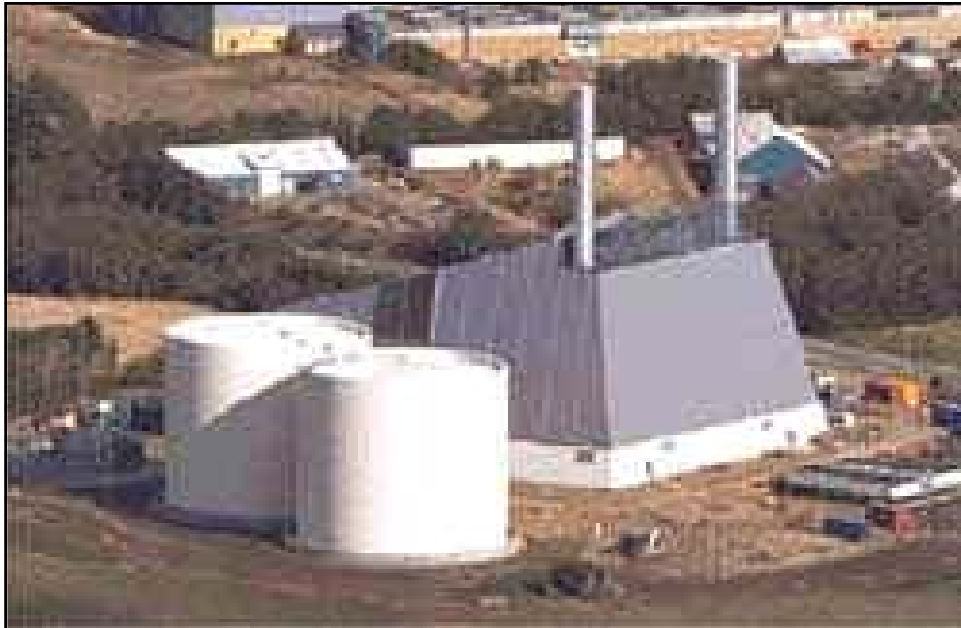
Picture of CHP unit with two heat accumulators (thermal stores) on left
