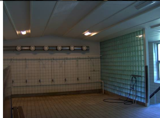
Bathing facilities in gymnasium.
