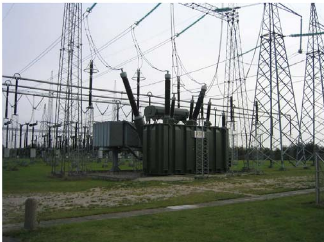
Fig. 3. A photograph of the 400/150 kV power transformer and its nearest surroundings
