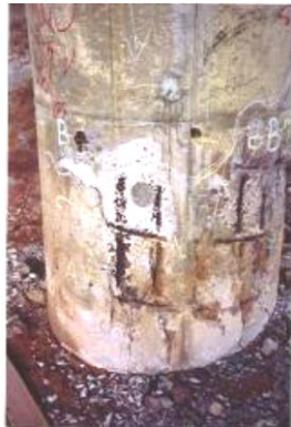
Figure 14. Corrosion cracking and spalling.
