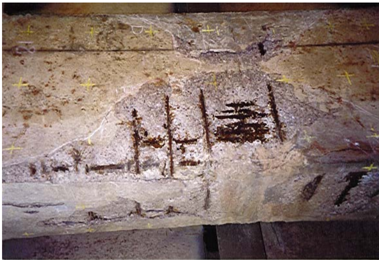
Figure 1. Corrosion cracking of a reinforced concrete beam.
