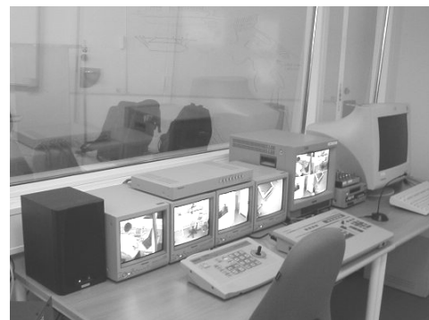
Figure 10. The control room
