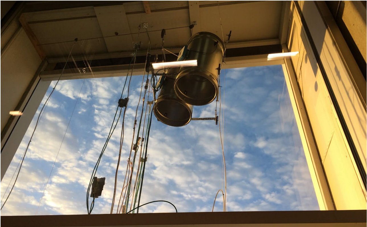
Figure 32: Internal view on the Ultralink air flow sensors (Lindab) in the ventilated cavity of the DSF 23 setup.
