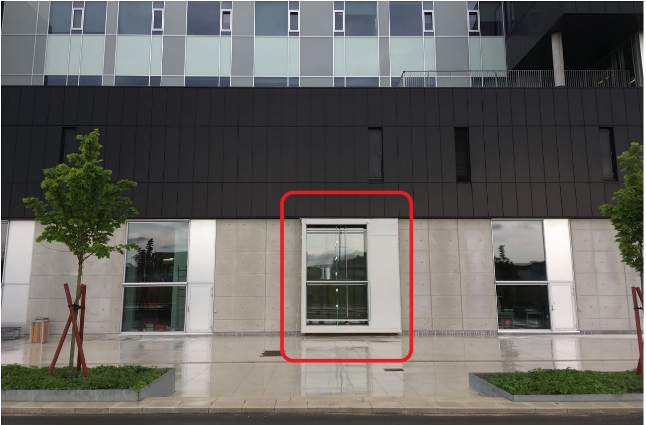
Figure 25: Front view of the DSF 23 experimental setup integrated into the south façade of the laboratory building at the Department of Civil Engineering of Aalborg University [1].
