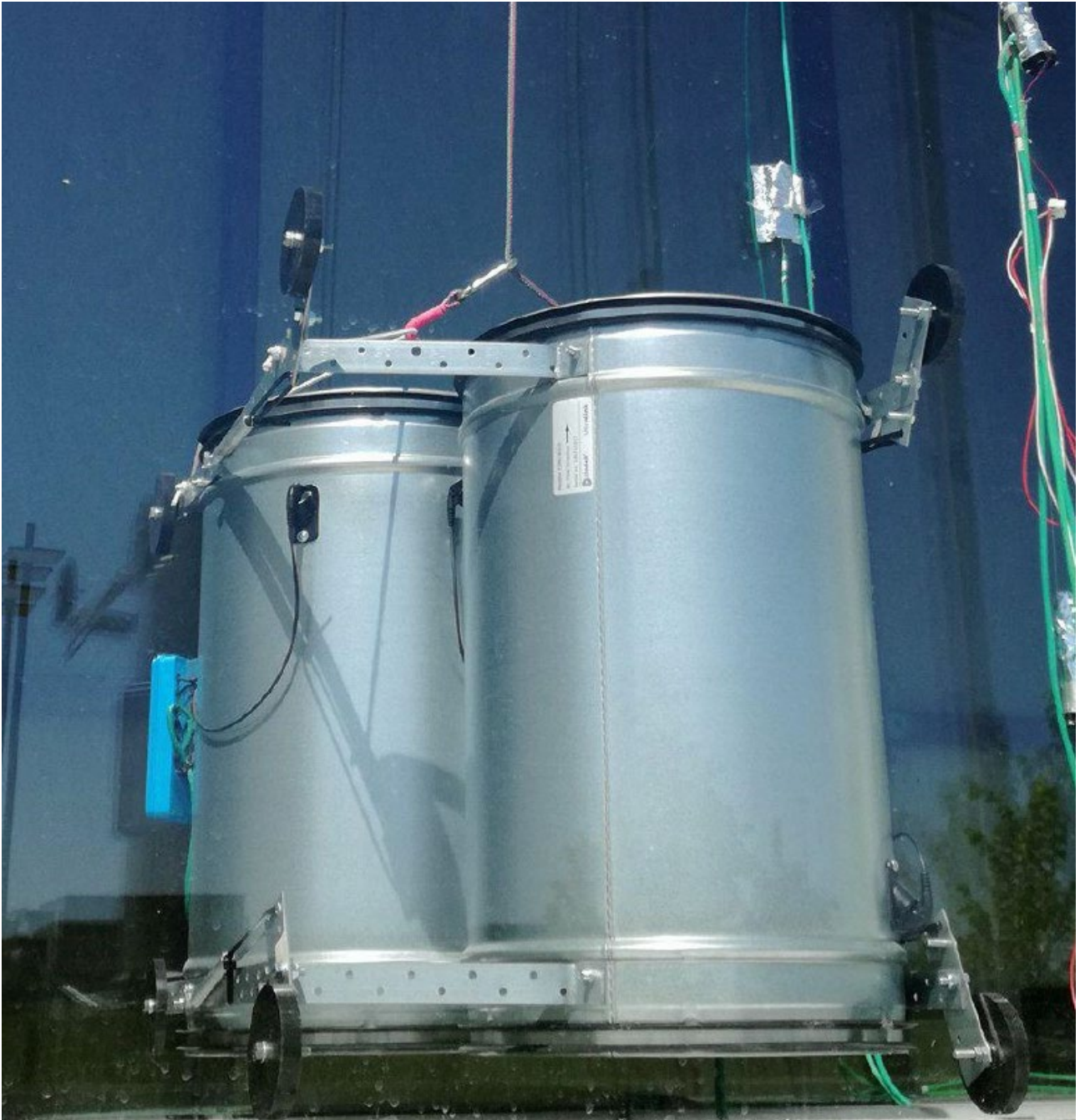
Figure 31: External view on the Ultralink air flow sensors (Lindab) in the ventilated cavity of the DSF 23 setup [1].
