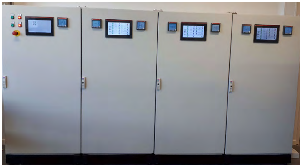
Figure 7 – The four control cabinets +A1...4 for the Microgrid Setup showing the ABB CP600 touch-panel and ABB M2M Digital Analysers.
