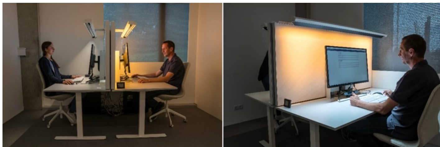
Figure 2: Left: A double workstation equipped with 2 PTLs with differently personalized settings. Right: Different lighting settings for the rear wall (2200 K) and the table (4000 K), © Bartenbach
