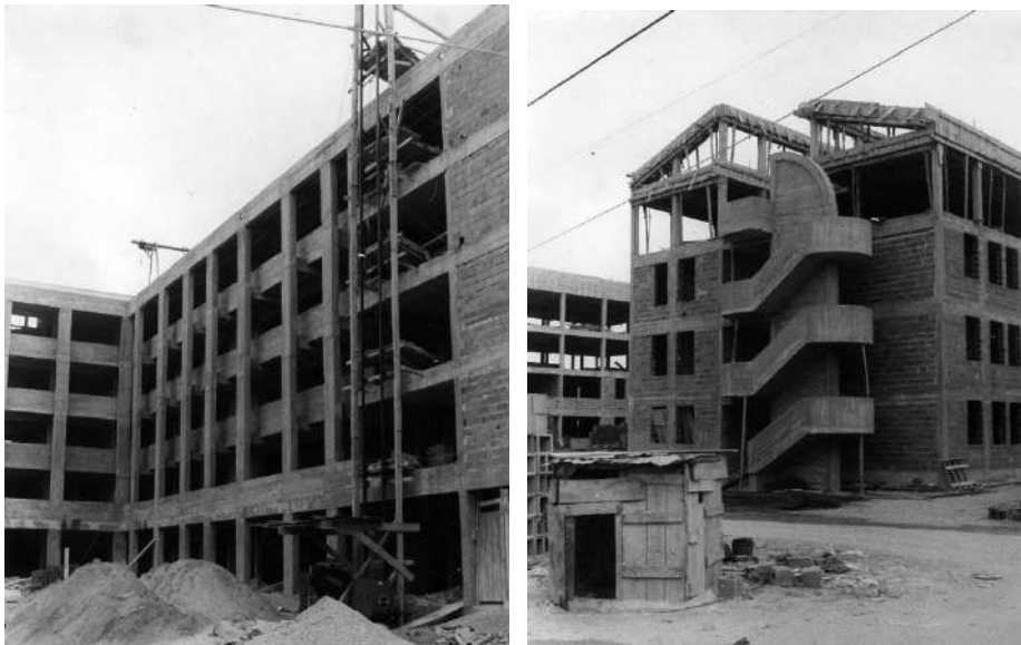
Fig. 15 - SAAL - Cooperative New Portugal: Architecture Project under construction. Photograph by Nuno Matos Silva, n.d. (ca. 1983)
