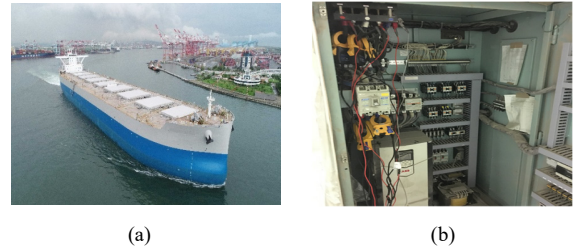
Fig. 6 Electrical power system of a bulk carrier ship. (a) Picture of the selected bulk carrier ship. (b) Sensors of the measurement devices that are connected to the main switchboard of the electrical power system.
