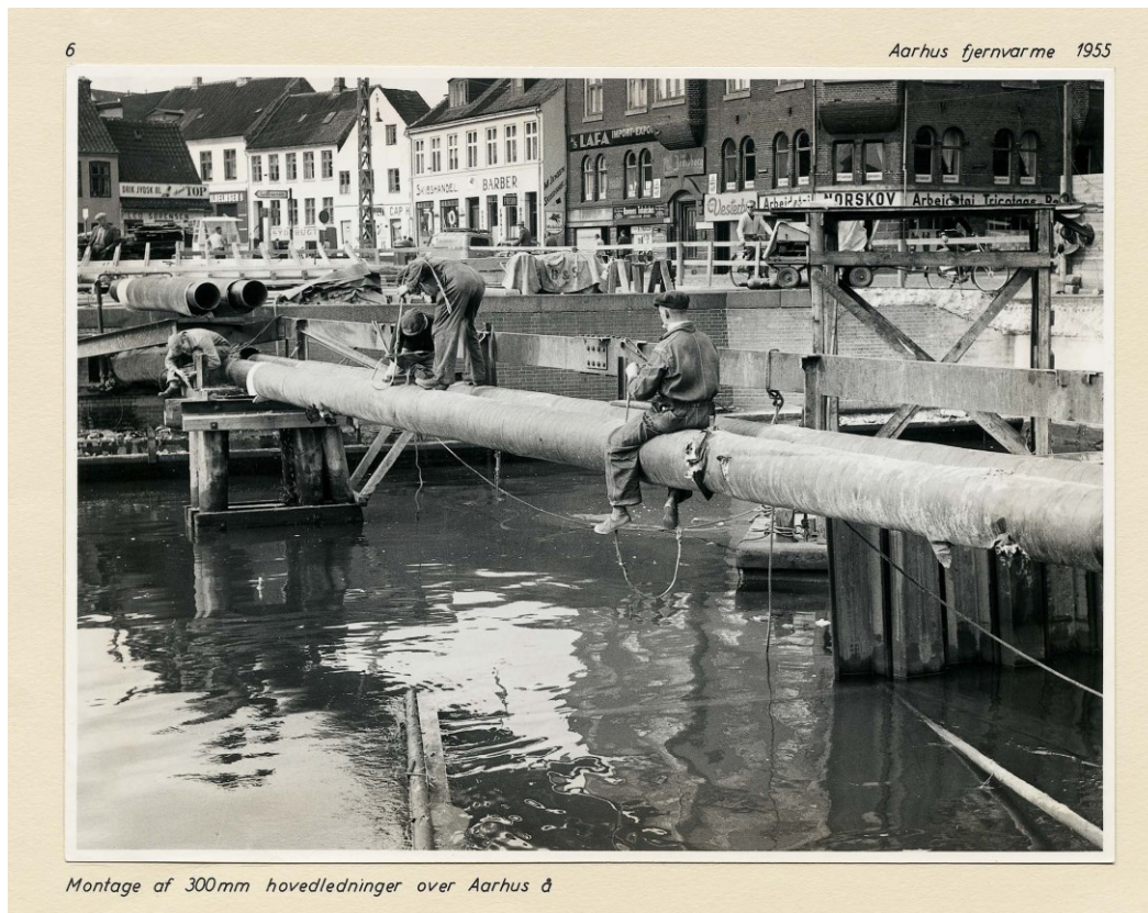
Figure 5: Installing 300 mm main pipes across Aarhus Creek, 1955. Printed with permission from Affaldvarme Århus
