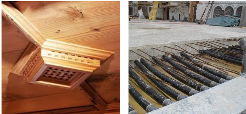
figure 4: left: supply air opening in a farmhouse in Tyrol © Michael Flach, right Ventilation pipes in the floor at Doragno Castle in Switzerland © L. Carugo
