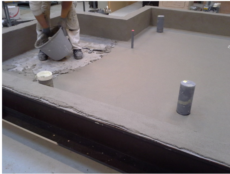
Figure 7. Mounting the test material inside the mock-up for System E, which is a two-component fixed mortar paste combined with edge reinforcements, epoxy and elastic pipe collars.
