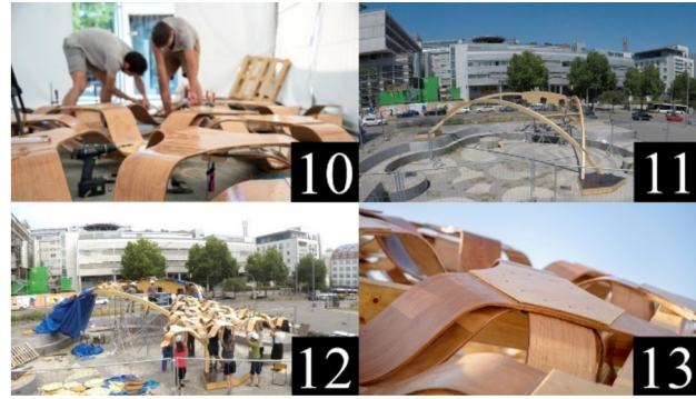
Figure 3: Assembly process and interconnection of sandwich panels (Source: © BioMat at ITKE/University of Stuttgart).
