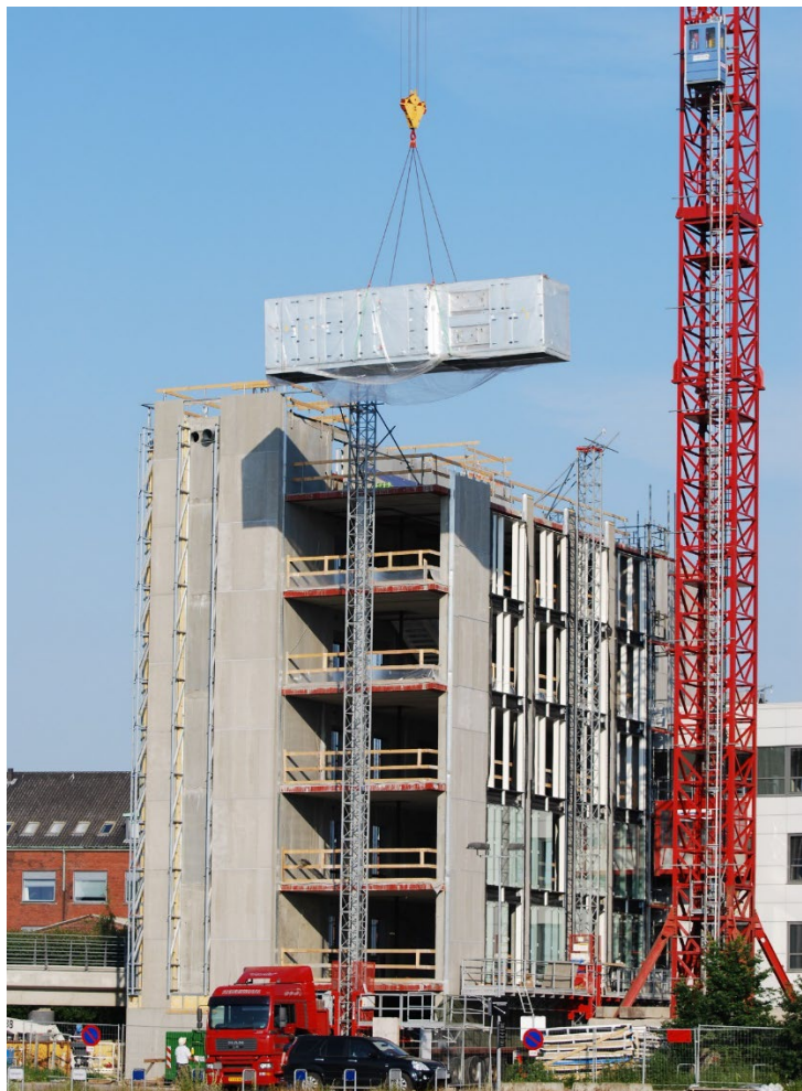
Figure 10: An IDCS unit being installed on the roof-top technical room of a new building (not the current test building project).
