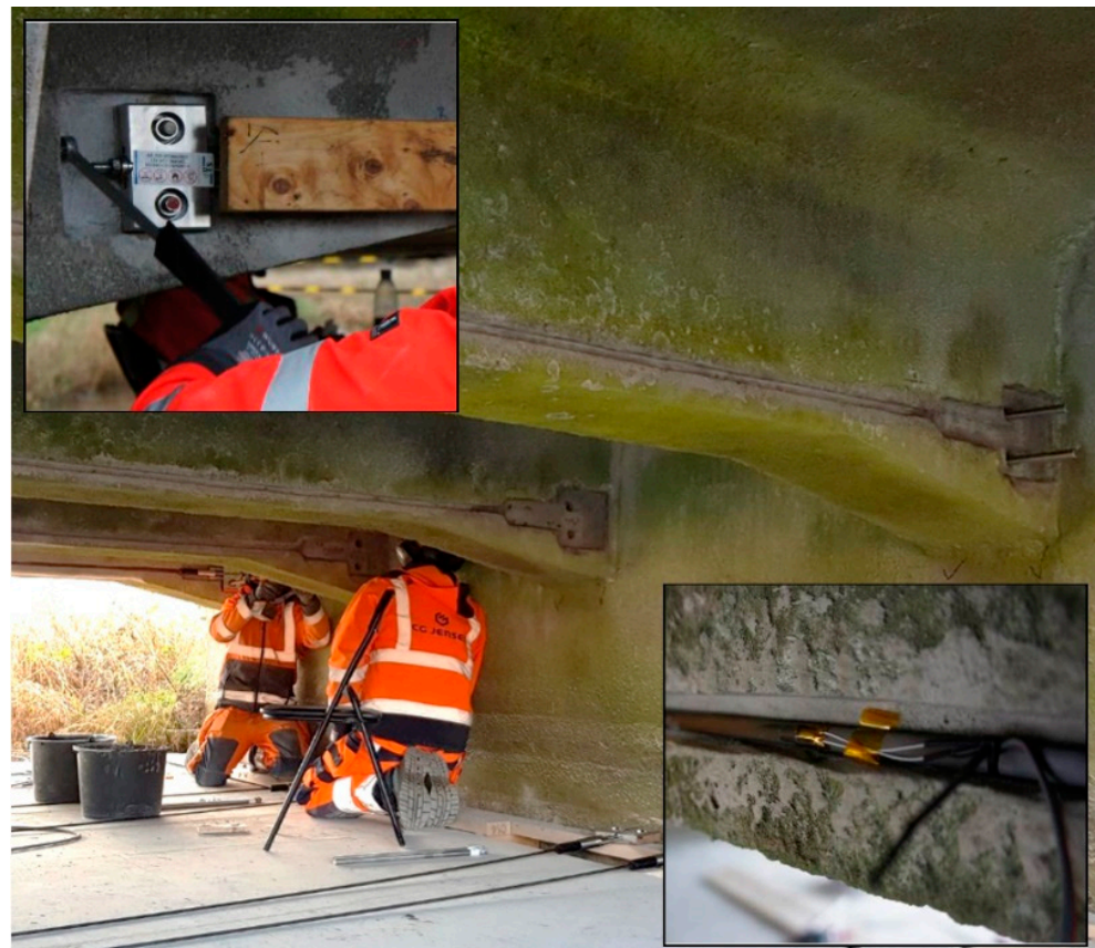
Figure 16. Site installation of the throughgoing threaded bar and pre-stressing of the system. Photograph by S&P.
