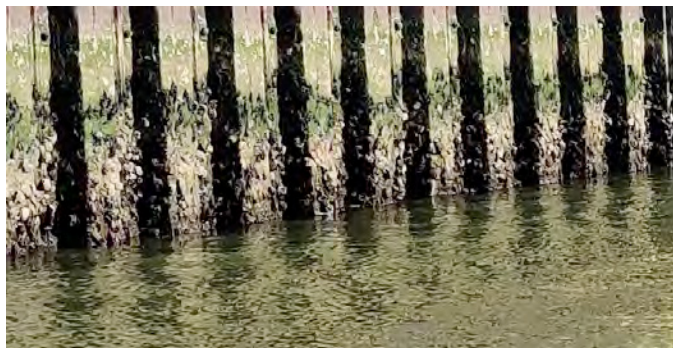
Fig. 8. Photo of the harbour wall at Port of Esberg above sea level where the sensor tests were conducted
