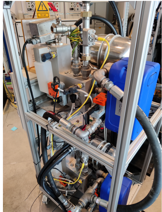
Fig. 7. Cooling system for LV and MV PECs.
