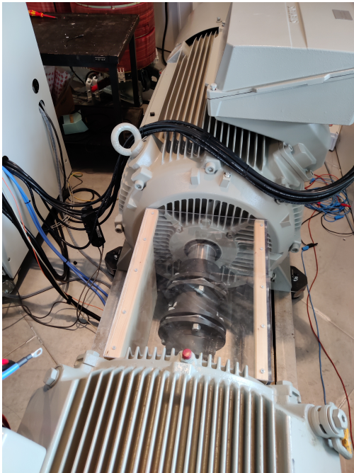
Fig. 4. LV and MV inductions machines mechanically coupled.
