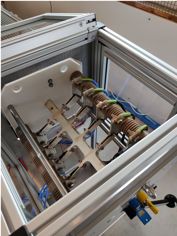
Fig. 6. Grounding switch; Shorts and grounds DC-links and high potential AC 3-phase lines.
