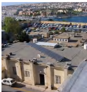
Photovoltaic panels installed on a government-owned building
