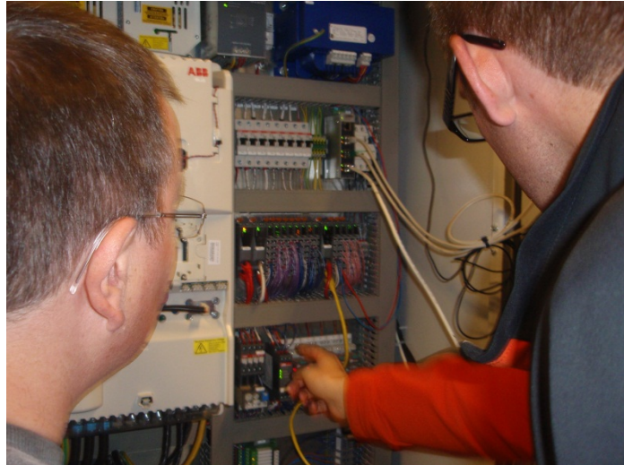
Figure 7.50: Regulation experts looking into the decanter's control cabinet searching for the reason why the connection isn't working. Picture By Author, fall 2011
