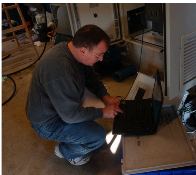
Figure 7.7: PLC expert kneeling in front of the control cabin while setting up the equipment he just brought. Picture by Author, fall 2011.
