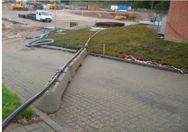
Figure 7.2: Hose supplying wastewater to the decanter shed. Picture by Author, fall 2011
