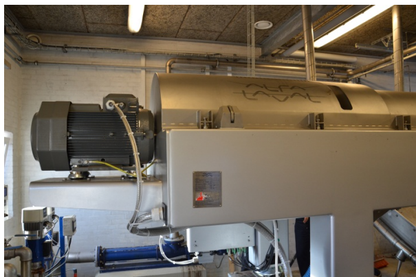
Figure 7.3: The decanter seen from the end that receives the wastewater. Behind us we have the control installations. Picture by Author, fall 2011.
