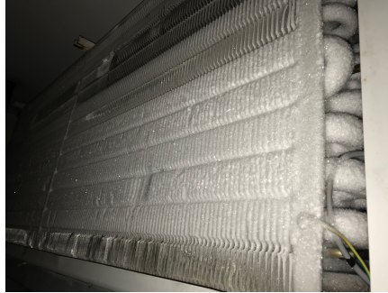
Fig. 25: The effect of evaporator fan fault on the evaporator of the laboratory setup at sample 17700 in Fig. 24. Papers A and B aim to detect the evaporator fan fault in the system before ice accumulates around the evaporator coil or cold room temperature becomes uneven. In this experiment defrosting mode of the system was off.
