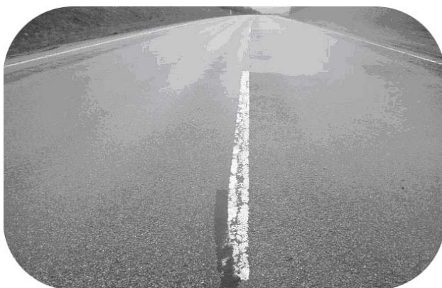
Figur 61. Slidt midterafstribning i km 0,47.
