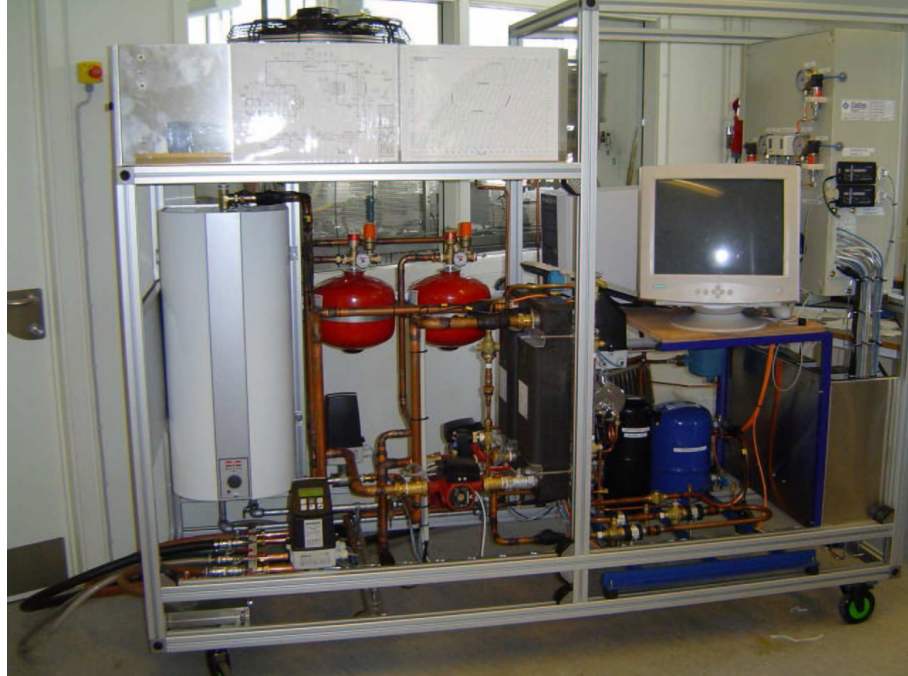
Figure A.1: Picture of the test refrigeration system
