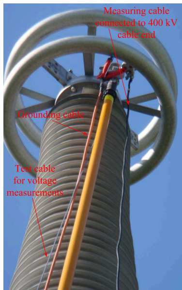
(a) The measuring cable.
